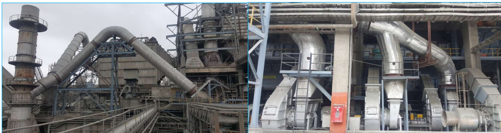
Duct From CV Stack
